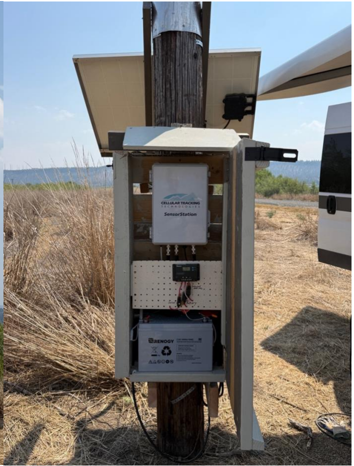
SensorStation with power supply and solar panel mounted on a pole
